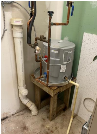
Figure 8: Existing electric water heater in mech room will be replaced with larger heat pump model.
