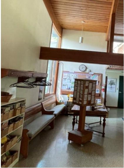
Figure 6: Lobby finned tube radiator under window to be replaced with CUH.
